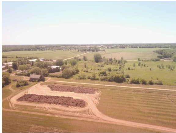
Stockpile of stumps and rocks pulled from the old tree lines running through the site (6/16/2021)
