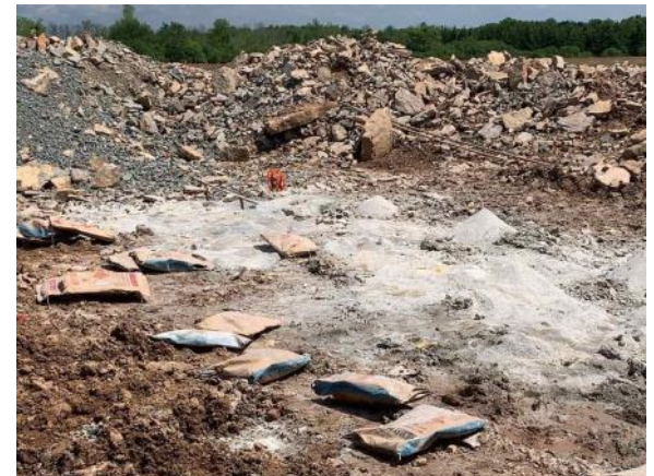
Many holes are drilled and filled with explosives for the rock blasting (6/30/2021)
